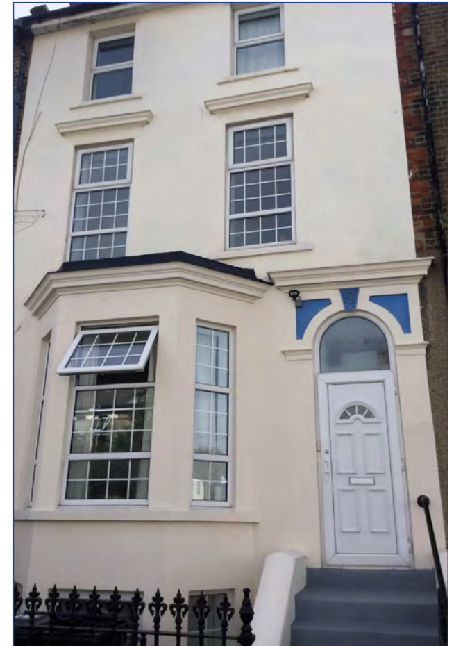
Well-intentioned unsympathetic changes to windows and doors have had a damaging effect on our conservation areas.
