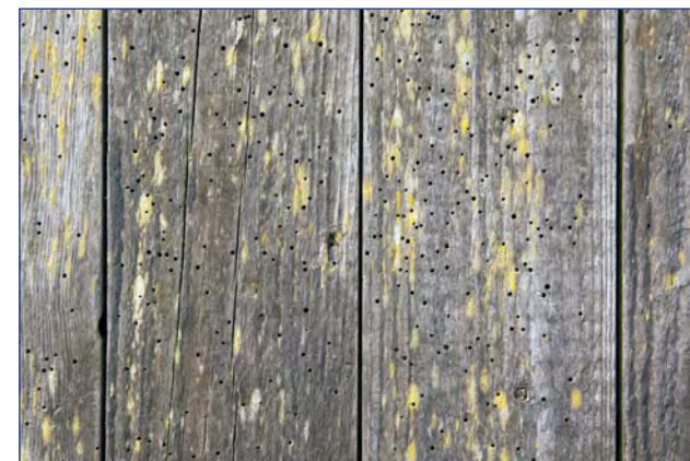
Evidence of wood boring insects does not necessarily mean you have a live infestation.
