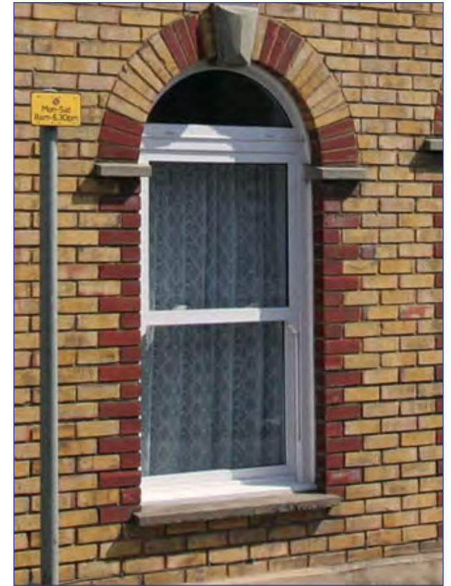
Replacement does not respect the shape and proportions of the original window opening and glazing bars.
