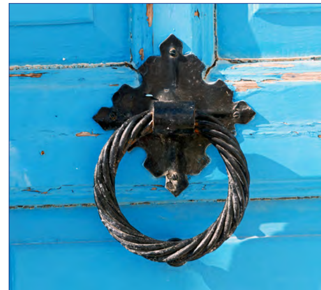
Exterior paint failure will allow moisture to penetrate timber.
